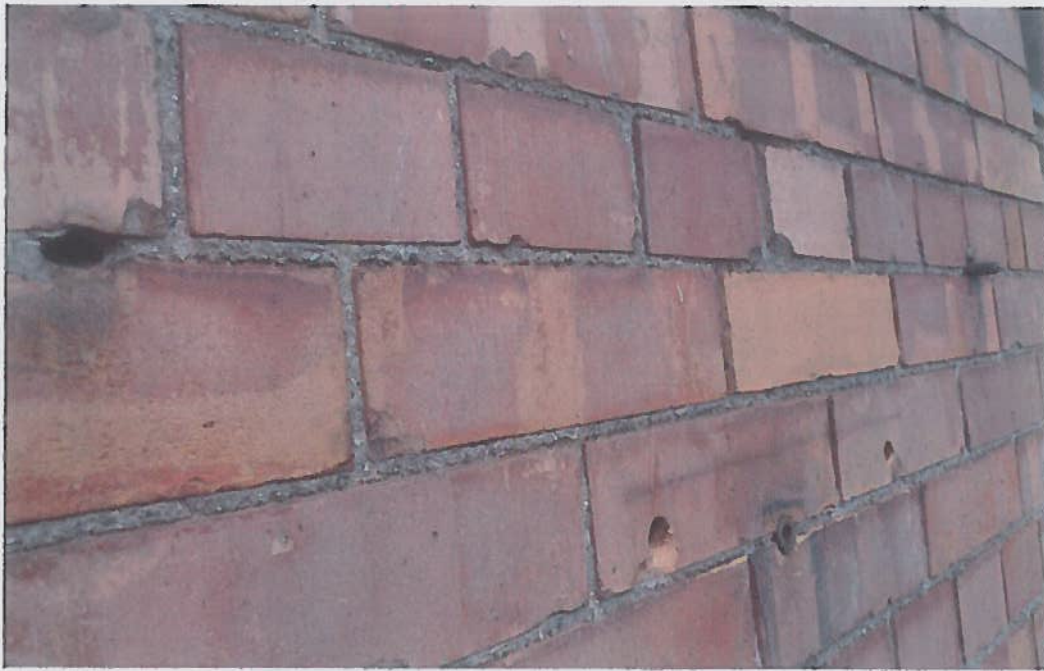
Photo 04 – Impact damage (possible bullet strikes) to bricks
