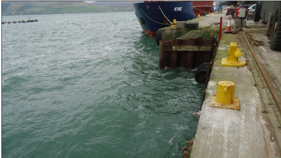
Plate 9: View looking towards the north end of Berth 2, showing it is recessed from the façade of Berth 1. In the proposed development, the new façade of Berth 2 will be flush with that of Berth 1, offering a continuous quay wall.
