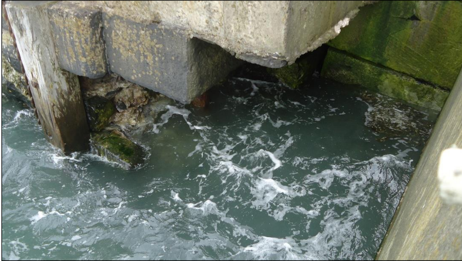
Plate 11: View at the south end of Berth 2, showing the base of the concrete deck than is placed on top of the stone-built quay. The picture also shows the scour that has developed at this junction, producing a large cavity.
