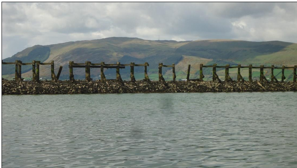
Plate 8: View looking north-northwest across central portion of the Breakwater feature to the west of the quayside, at Low Water. The solid rock-armoured base supports an open-work lattice of concrete members that are exposed at High Water, and may have held a deck in former times.
