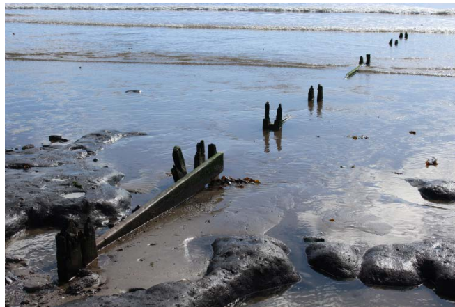
Figure 4 Dilapidated timber groyne on the foreshore
