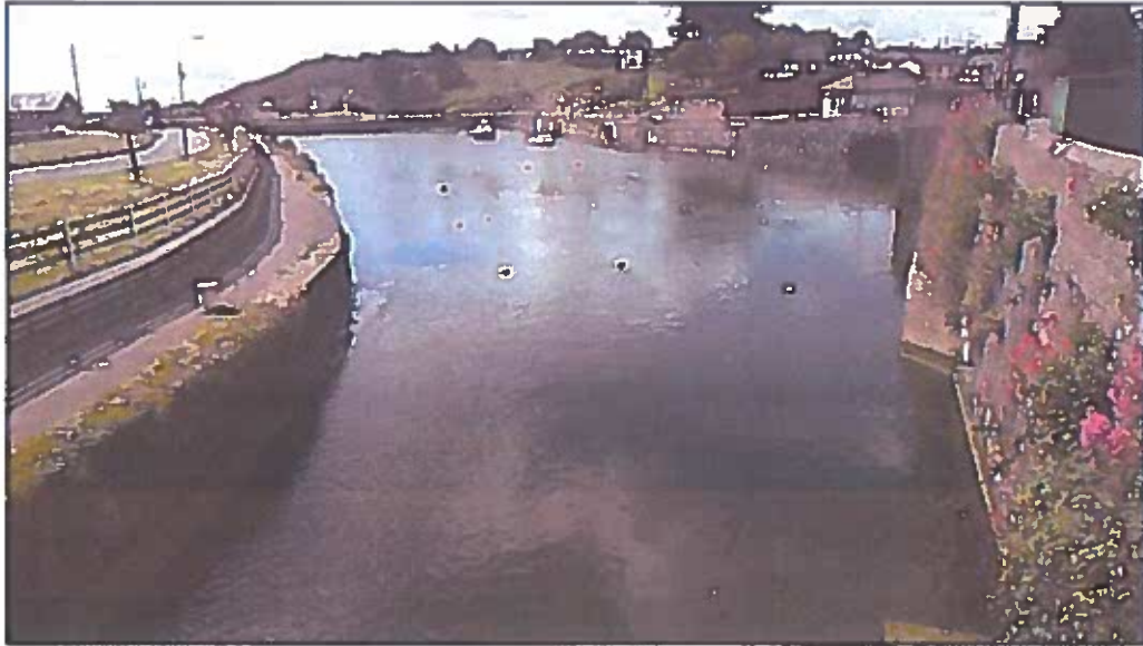
Plate 10: View looking south into the larger basin, highlighting the concrete lintels that run along the base of the quay walls.
