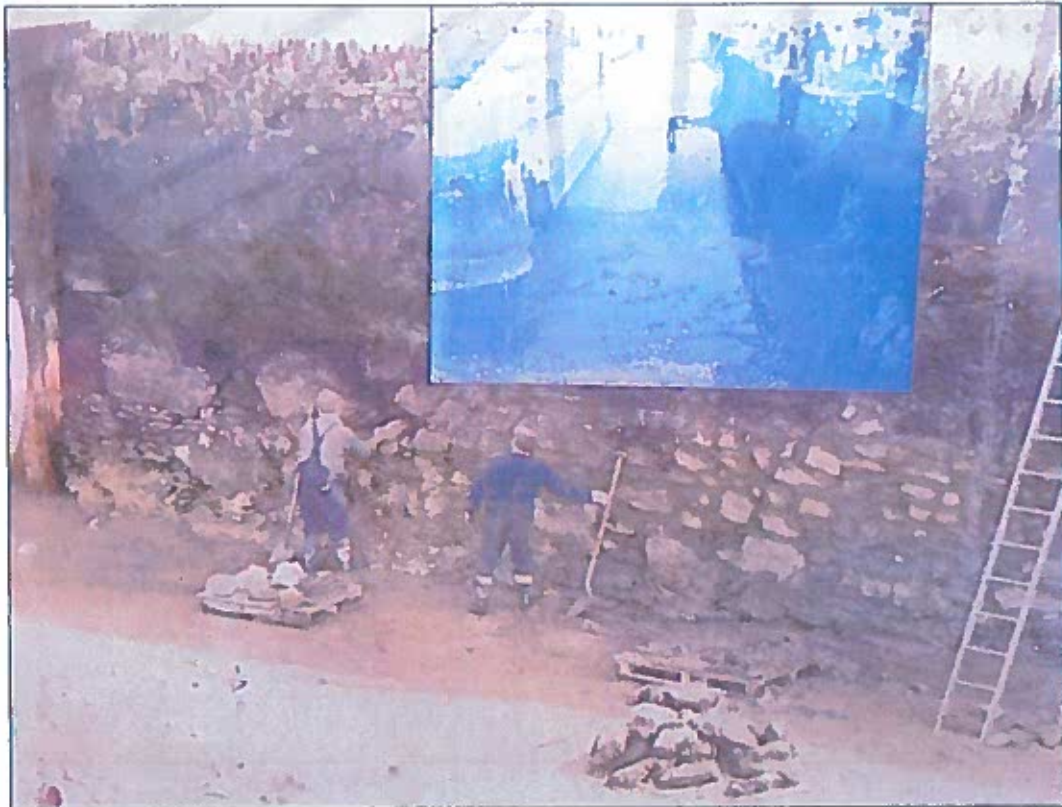
Plate 14: Detail from 1980s' photograph showing repair work to quayside stonework while the basin was drained. Source: Tara View Hotel.
