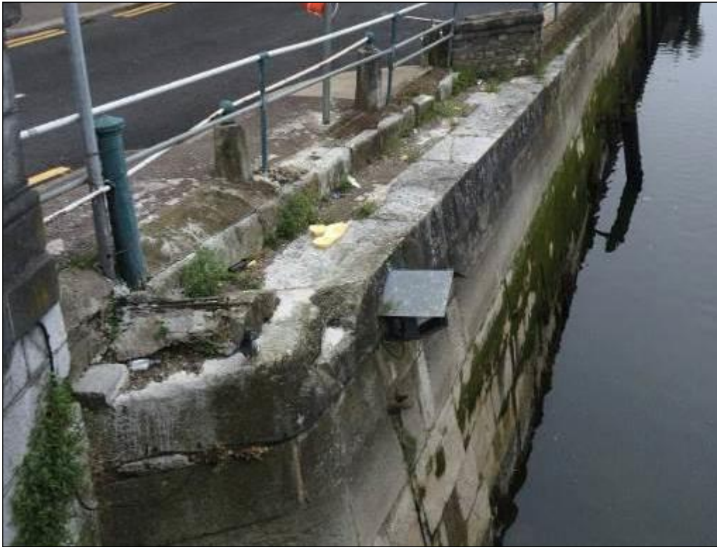
Plate 10.6: View of surviving section of railing at west end of Father Mathew Quay (HAN 1) from west. A small section of modern walling has been inserted into a railing gap at the east end of the bollards
