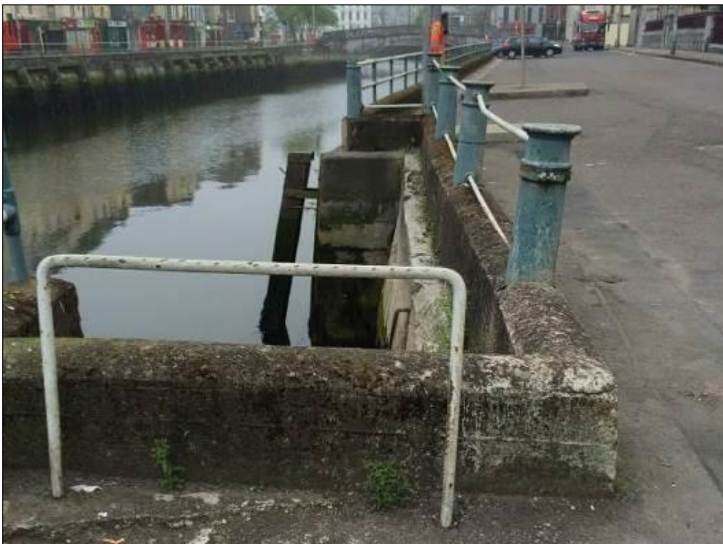
Plate 10.12: View of bollards extending around Father Matthew Quay steps from east (HAN 1). These have been incorporated into the modern railing concrete base and it is unclear whether they were left in situ while this feature was installed or if they were removed and then reset afterwards
