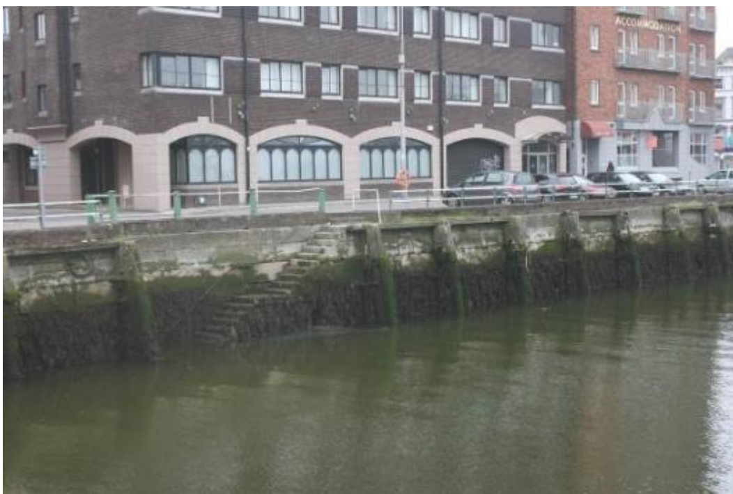
Plate 10.17: View from southwest towards western steps and side rail on Morrison's Quay (HAN 2). A mooring ring is also visible along the top of the section of quay wall to the left
