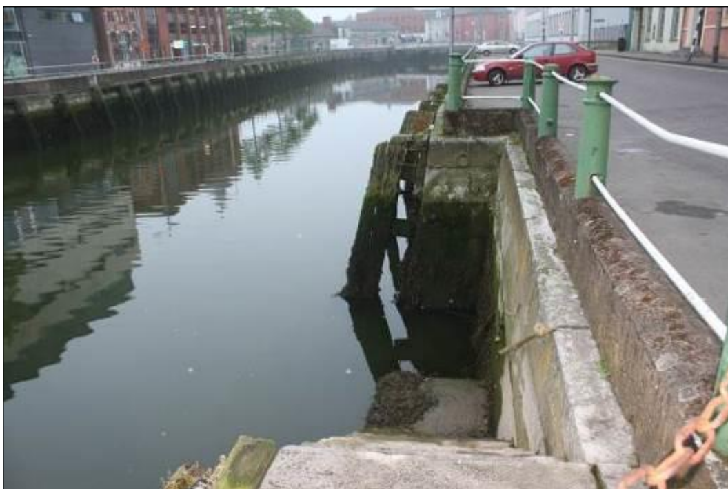
Plate 10.19: View from east towards western steps on Morrison's Quay (HAN 2) with a small mooring ring visible on the opposite wall section
