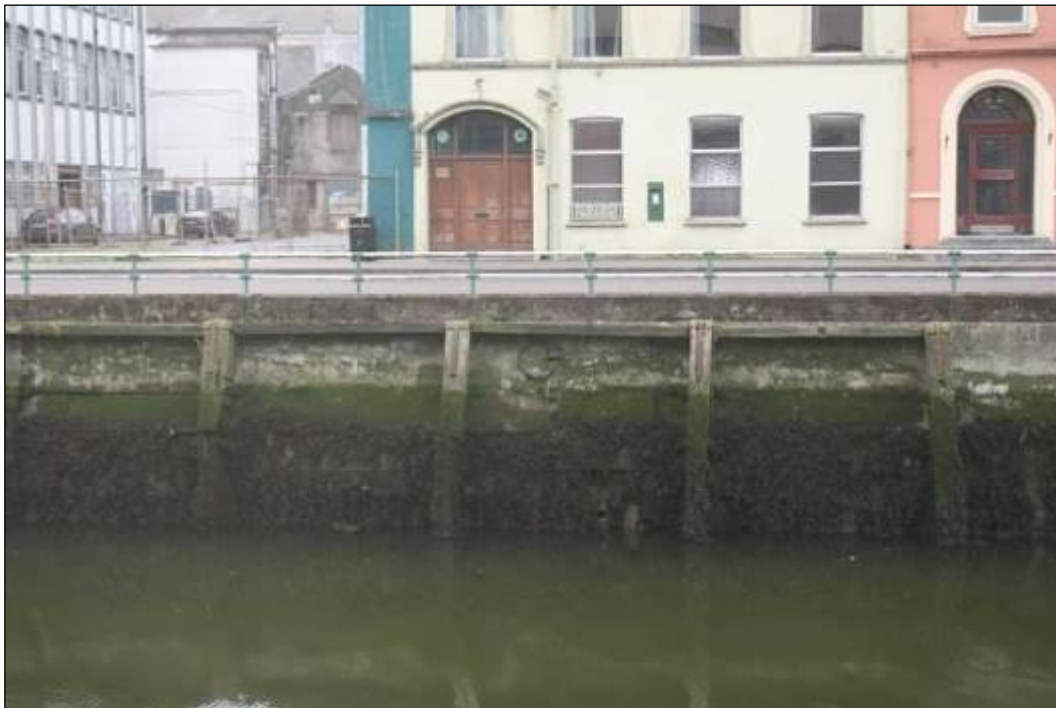
Plate 10.16: View of elevation of Morrison's Quay wall (HAN 2) showing fenders and modern railings. An example of one of the mooring rings set into the wall is visible near centre of the photograph and the Assembly Rooms and associated post-box (HAN 13 and 12 ) are visible in the background
