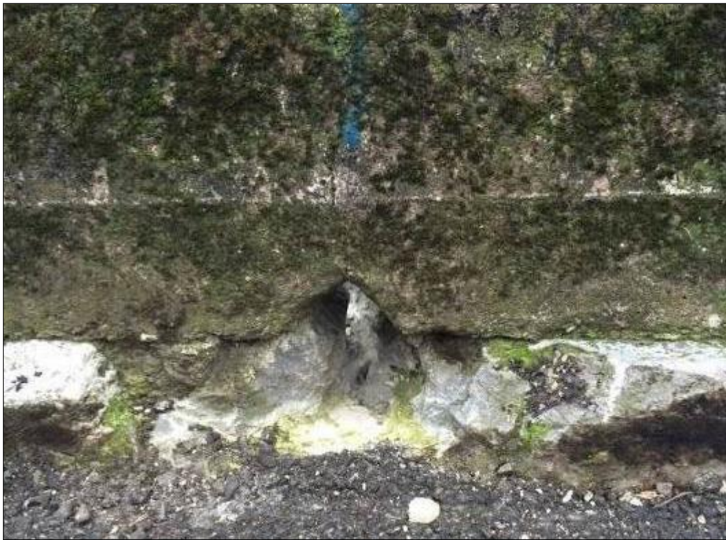
Plate 10.9: View of rough break recently inserted into upper course of Father Matthew quay wall (HAN 1), perhaps to facilitate drainage of rainwater
