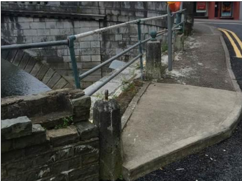
Plate 10.7: View of surviving bollards at west end of Father Mathew Quay (HAN 1) from east with Parliament Bridge (HAN 4) in background. These have been incorporated into a modern pathway and tarmac from recent road surface works directly abuts the easternmost example.
