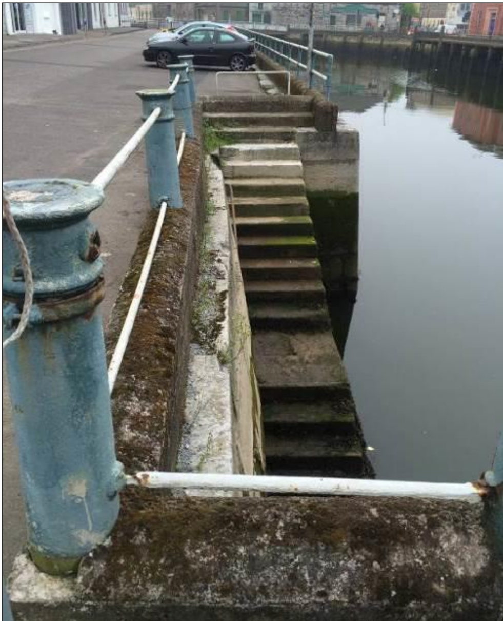
Plate 10.13: View of quay steps from west showing side rail inserted into Father Matthew quay wall (HAN 1) and sections of repair to upper steps with both limestone and concrete insertions. Traces of modern repairs to the quay walls are also visible, e.g. upper course to right of steps.
