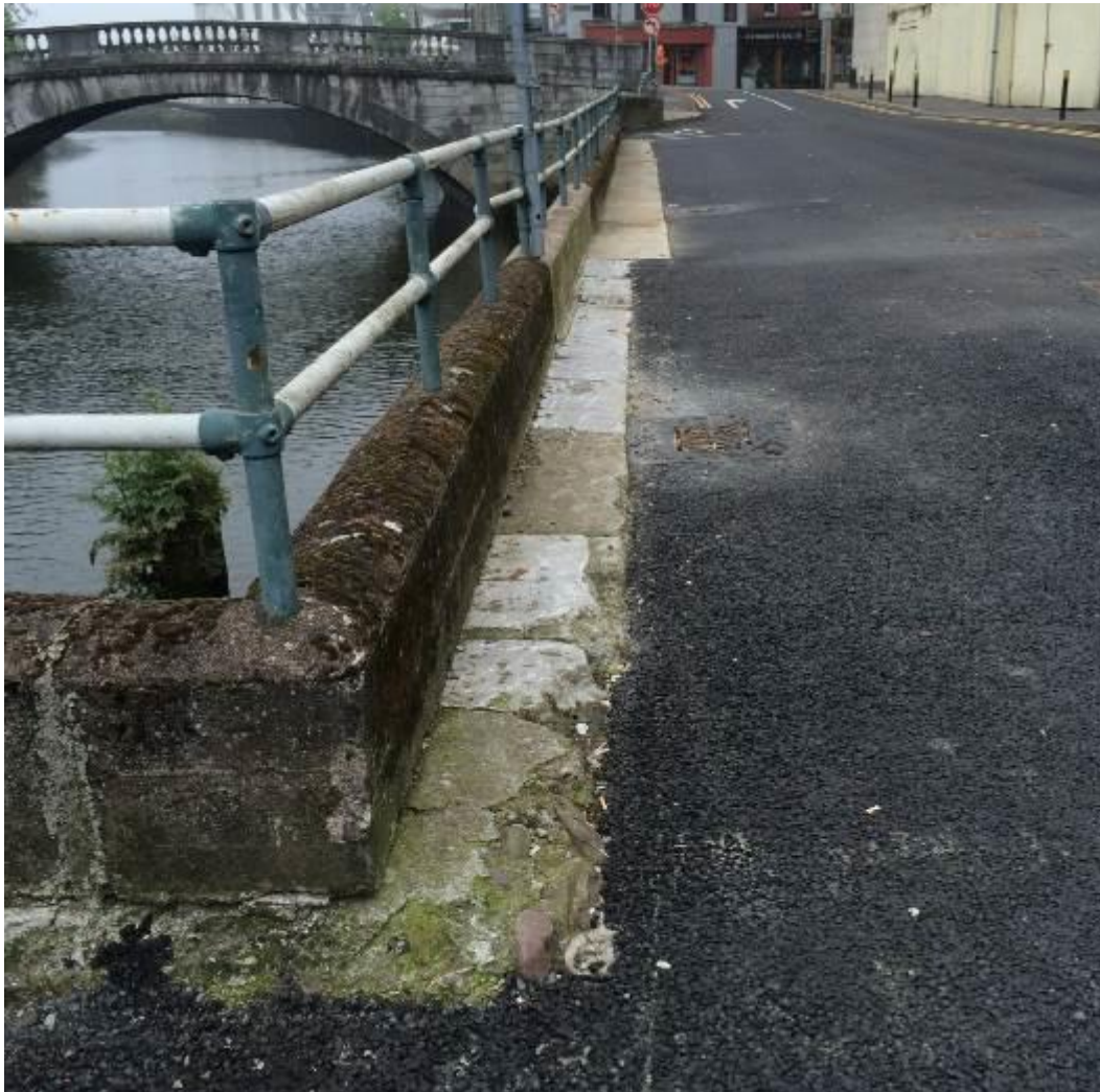
Plate 10.8: View of modern railings and concrete base along west end of Father Matthew Quay (HAN 1). Sections of damage and repairs to upper course of quay wall are also visible. The section of the adjacent road was subject to re-surfacing works in 2015
