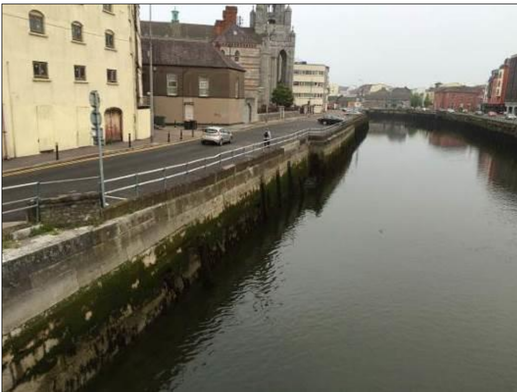
Plate 10.3: General view of Father Mathew Quay (HAN 1) from west (taken from Trinity Bridge). The quay walls along Father Mathew Quay were subject to City Council remedial works that included repointing, grouting and support works (Evening Echo May 29, 2012).
