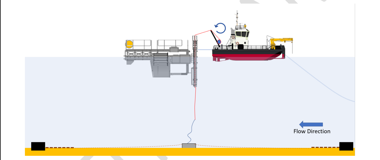
Installation vessel pulls up mooring system on winch, (expected lift force 7T).
