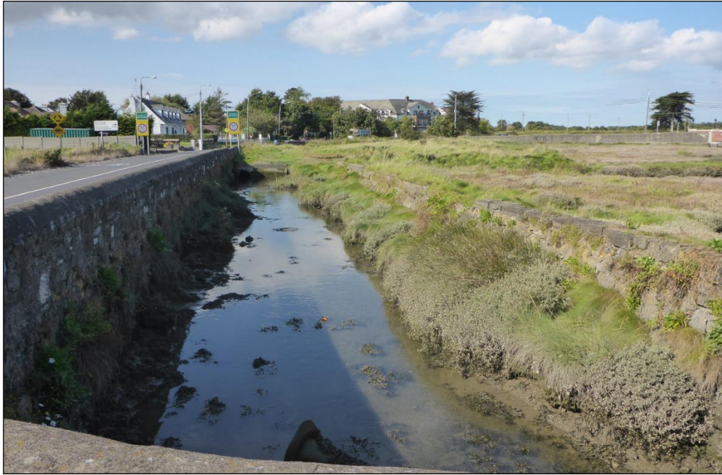
Plate 8 View looking northwest along the millrace channel, north of proposed storm water outfall pipe
