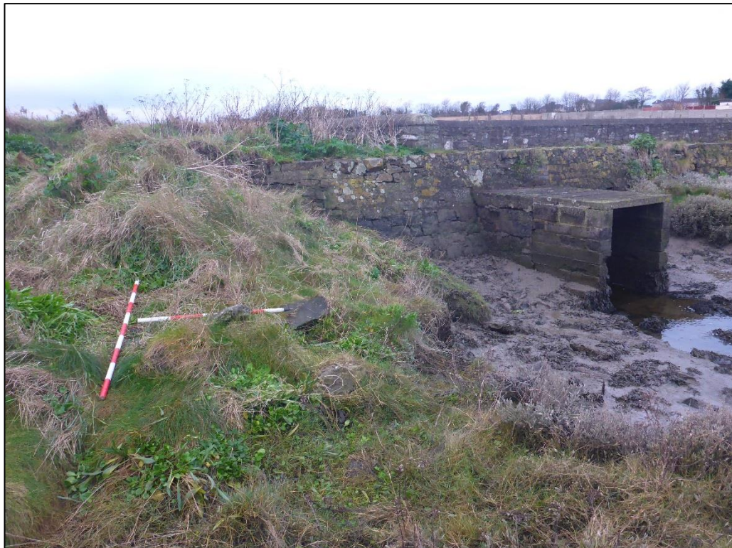
Plate 17 View of rubble stone blocks with the culvert/slucice gate in the background
