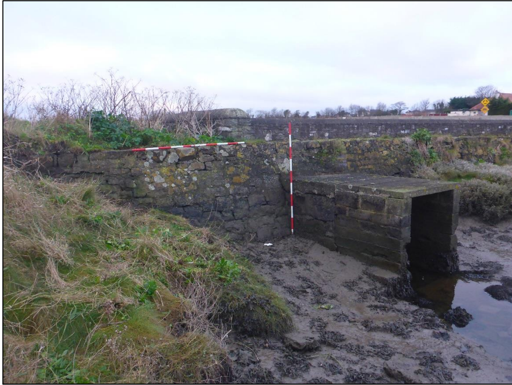
Plate 10 The stone and modern cement culvert located to the north of the proposed outfall works
