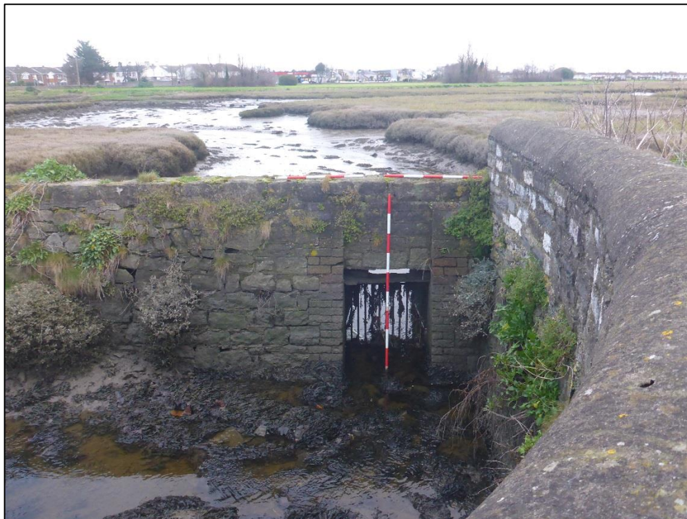
Plate 9 Sluice/ flood gate, located to the north of the proposed outfall works
