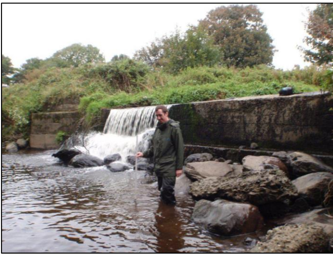
Plate 5.1. The confluence of the Rivers Moyvane and Galey, indicating the extent of excavation and deepening in the latter
