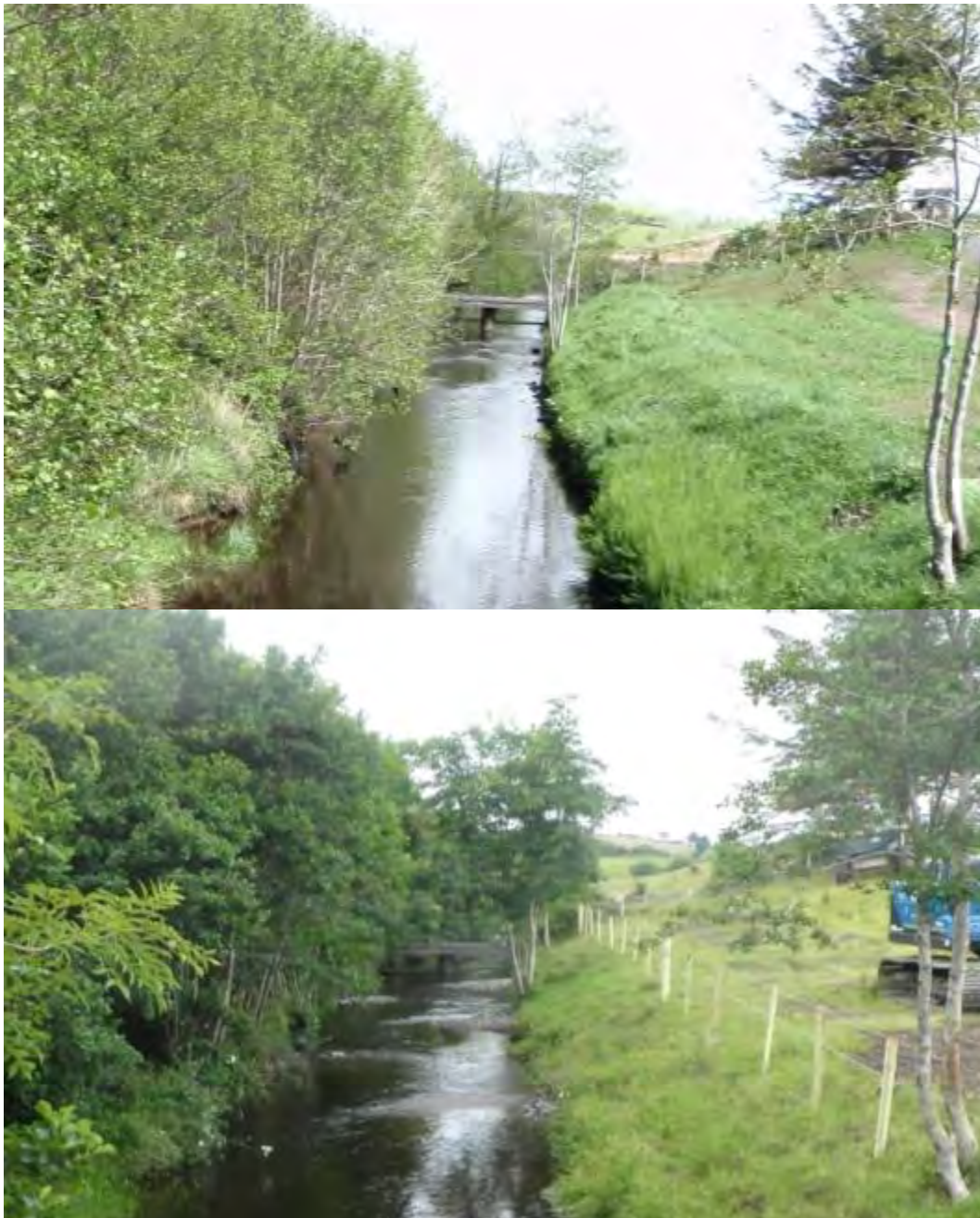
Figure 4.6. Constructed in 2016 experimental site 2 consists of a series of alternating deflectors (Top Pre works: 2014, Bottom immediately Post works: 2016) (note: OPW machine still on site)
