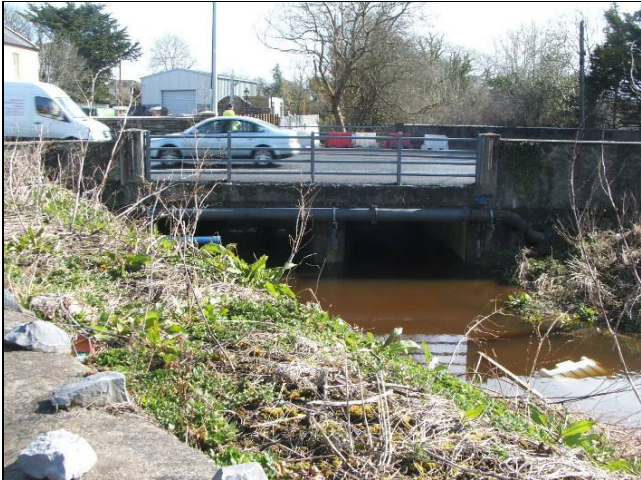
Photograph No. 4 N6 Bridge along the Bypass Channel looking upstream towards the channel shown in Photograph No. 1
