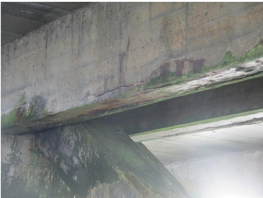
Photo 6 – Typical high-level beam delamination crack.
