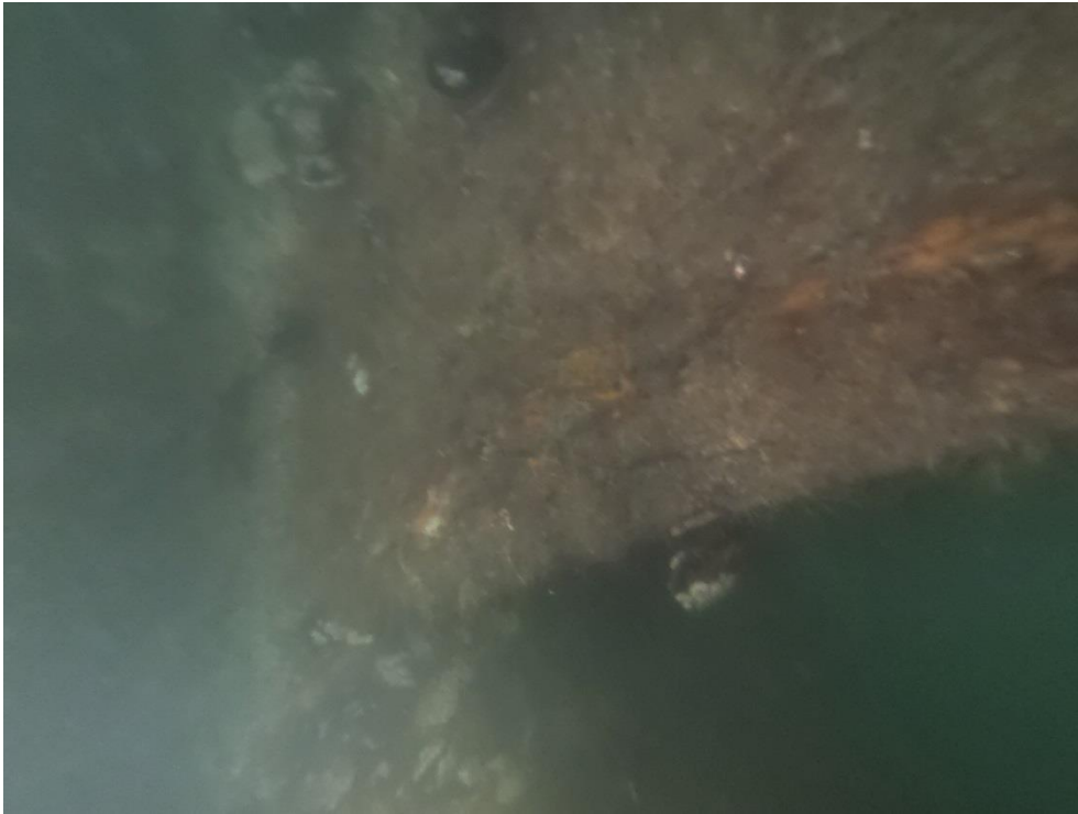
Fig B11 - Typical Delamination crack to bottom corners of VDM
