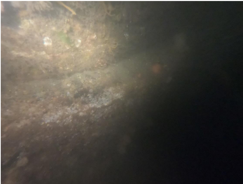
Fig B16 - Larger Diameter section exposed at base of column P18
