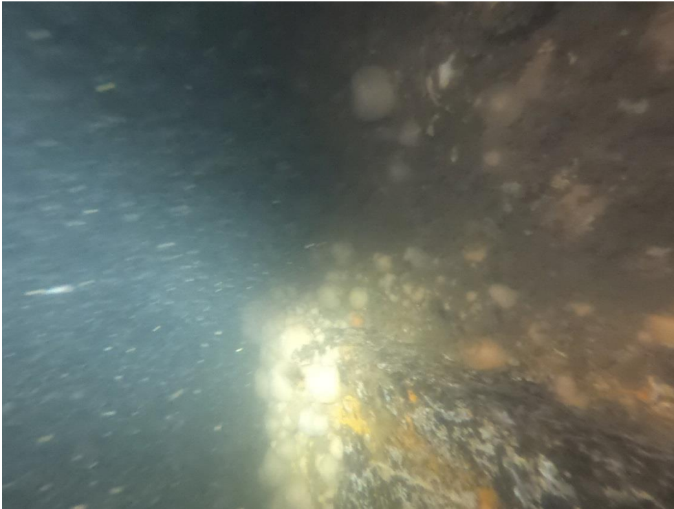
Fig B15 - Loss of section between pours – Column P19
