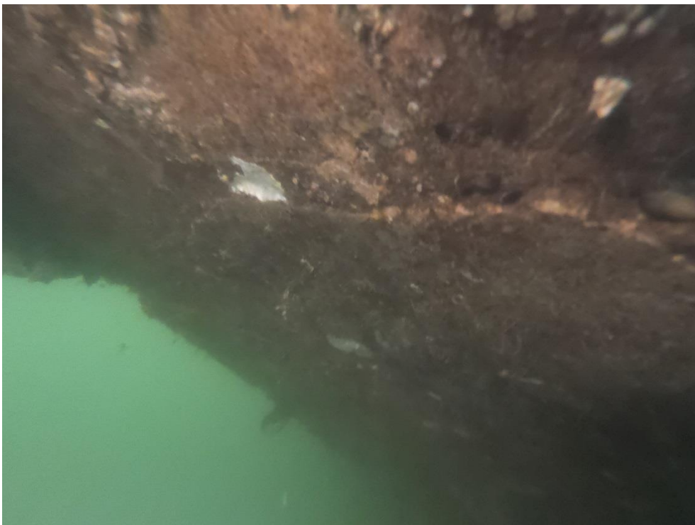
Fig B12 - Blown concrete to underside of VDM
