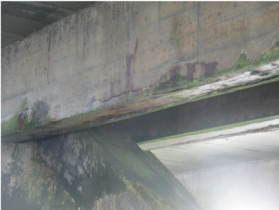
Fig B20 - Typical high-level beam delamination crack.
