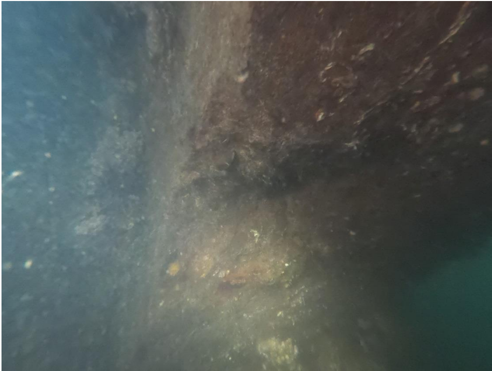
Fig B13 - Loss of concrete to underside of VDM (Frame 20)
