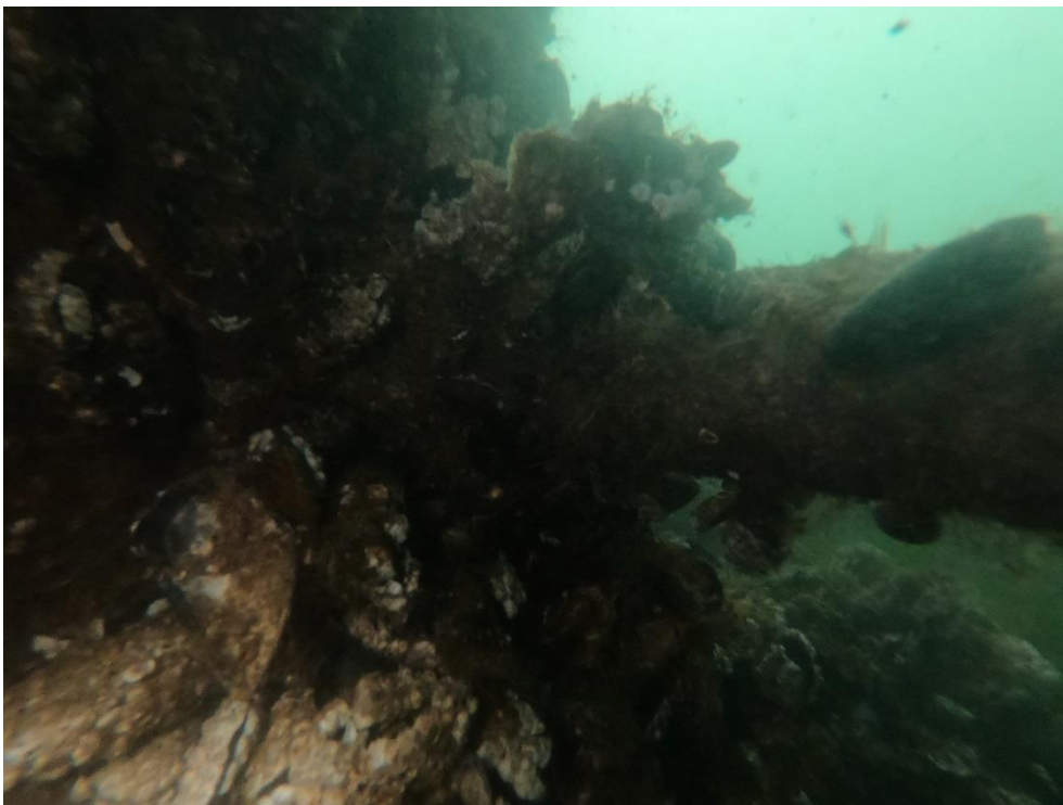
Fig B14 - Tie Bar protruding from column P22
