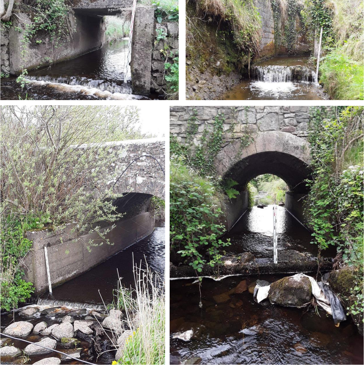
Figure 2.18 Bridge aprons with minor drops in the Breedoge catchment. Bella River (C6/4, top left); upstream tributary (C6/7/5/5); Mantua River (C6/9, bottom left); Owennafreesha River (C6/7/5 bottom right).
