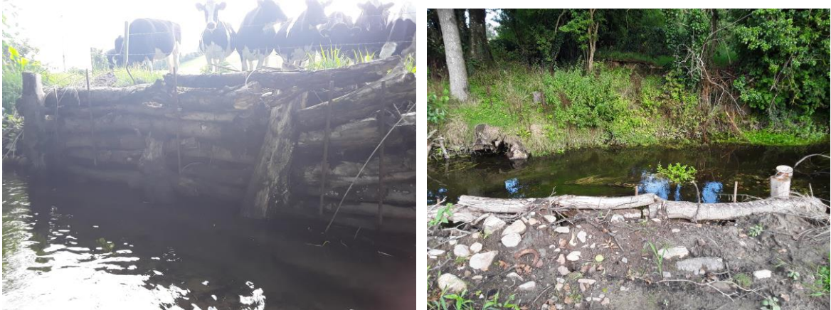
Figure 4.8 Woody bundle as bank protection (left – photo taken from the channel channel; right – photo taken on right-hand bank)
