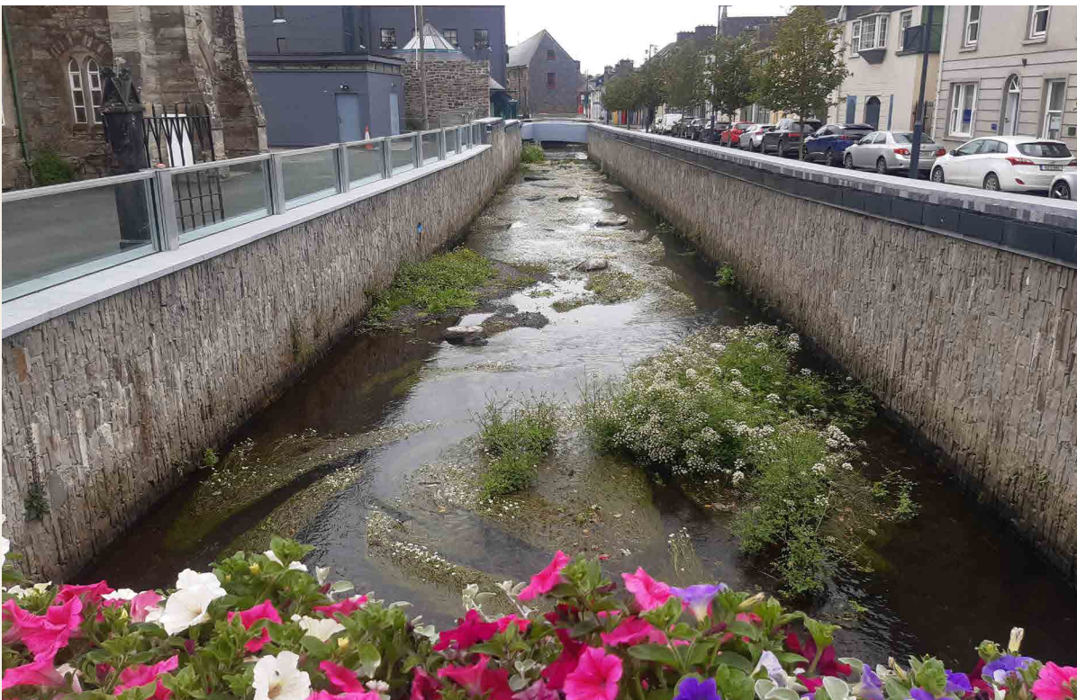
Clonakilty Flood Relief Scheme. Winner of the Innovation Category – Large Projects, ACEI Engineering Excellence Awards 2022
