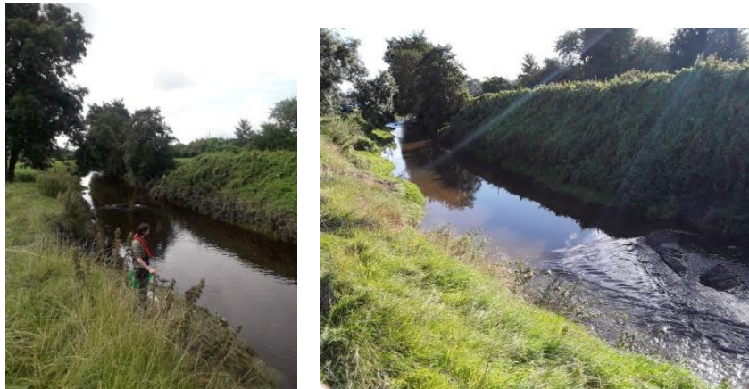
Figure 5.11 Left photo was taken pre-works showing a uniform glide and the photo on the right taken post-works. Changes in flows are evident following the introduction of paired deflectors which were created using the material from within the channel.
