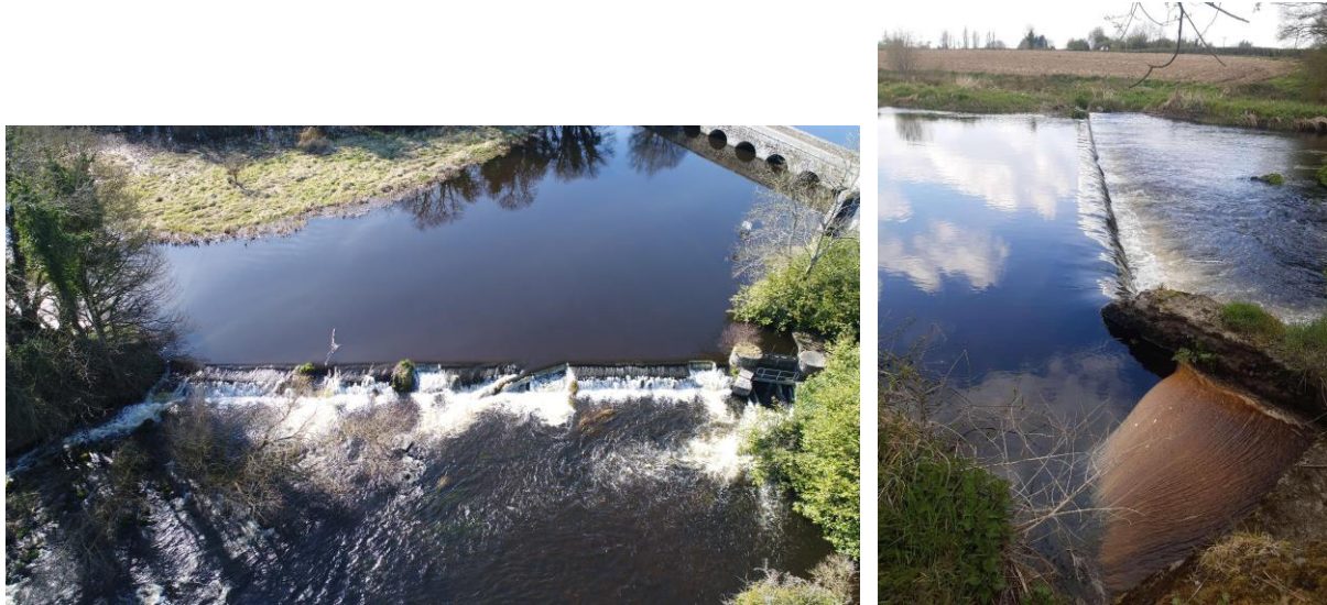
Figure 2.24 Headfort weir with a sloping face and central sloped fish pass (left) and abstraction weir at Clavens bridge (right).
