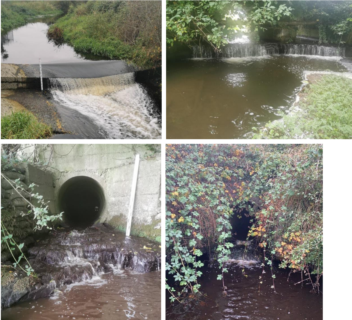
Figure 2.21 Small gauging weir (top left, C1/8/10); two-eye bridge with drop (top right, C1/8/15); culvert with apron and drop (bottom left, C1/8/16); perched culvert (bottom right, C1/8/19).
