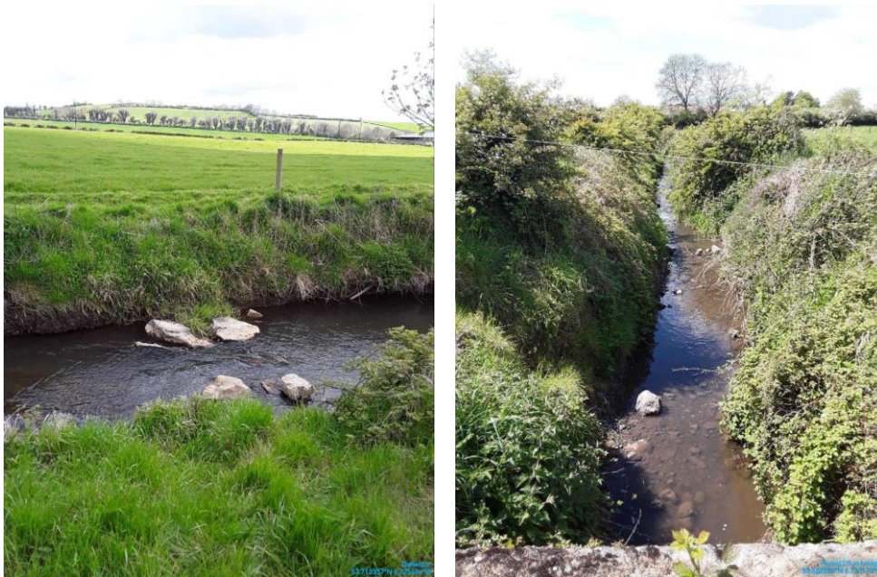
Figure 2.17 Artificial deflectors (left) creating good flows in a straightened part of the river channel C1/8/5 (Good status). Picture shows excessive silt on substrate (right), extensive over-deepening of the channel and simple native bank vegetation colonising the banks in channel C1/8/1 (Poor status).
