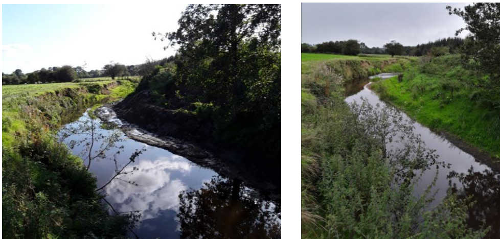
Figure 5.12 Left photo was taken post works of a berm topped during the works and the follow up photo on the right was taken in 2021.
