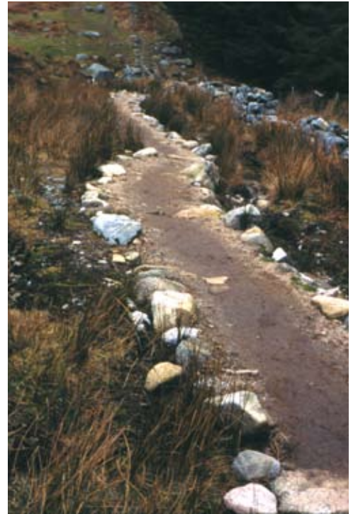
A well-constructed footpath will require less repair and maintenance, and represents a most sustainable solution in the long run. Djouce Forest, Co. Wicklow.
