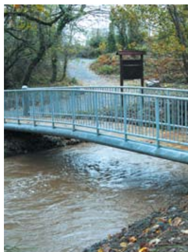
Complex and expensive bridging may be required to cross larger waterways in heavily used forests. Ballyseedy Wood, Co. Kerry.
