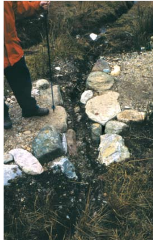
Waterbars, culverts and other drainage measures are a vital element of footpath construction. Djouce Forest, Co. Wicklow.
