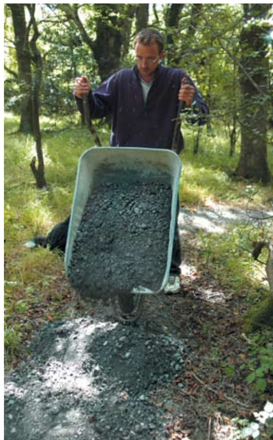
Incorporate the need for maintenance and repair when planning for recreation in the forest. Fairymount Farm, Co. Tipperary.
