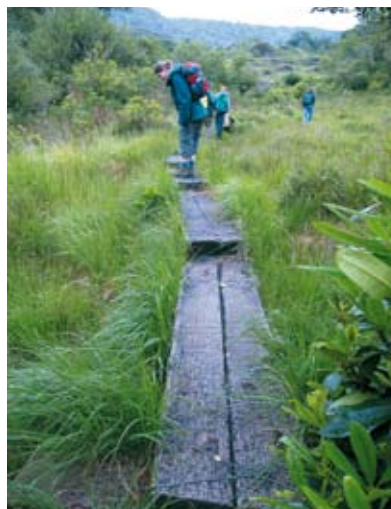
A simple boardwalk provides access across localised areas of wet terrain. Note the use of wire gauze for grip underfoot. Killarney, Co. Kerry. (Photo S. Bosbeer)
