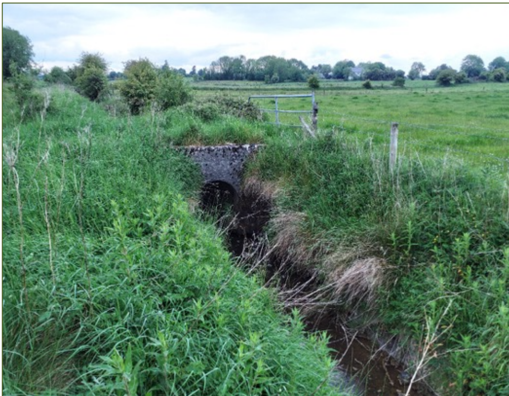
Plate 4.2: Bridge structure UB6 on Channel C3/26/5 (FW4) from the upstream side of the bridge culvert showing improved agricultural / wet grassland on either side of the channel.
