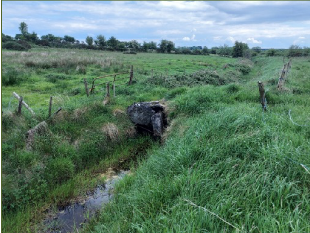
Plate 4.1: Bridge structure UB2 on Channel C3/26/5 (FW4) from the upstream side of the bridge culvert showing improved agricultural / wet grassland on either side of the channel.
