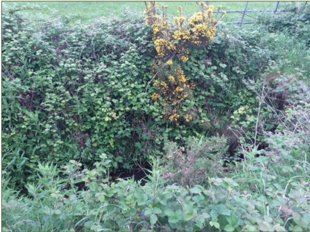
Plate 4.3: Bridge structure UB10 on Channel C3/26/5 (FW4) from the upstream side of the bridge culvert which is particularly overgrown with vegetation.
