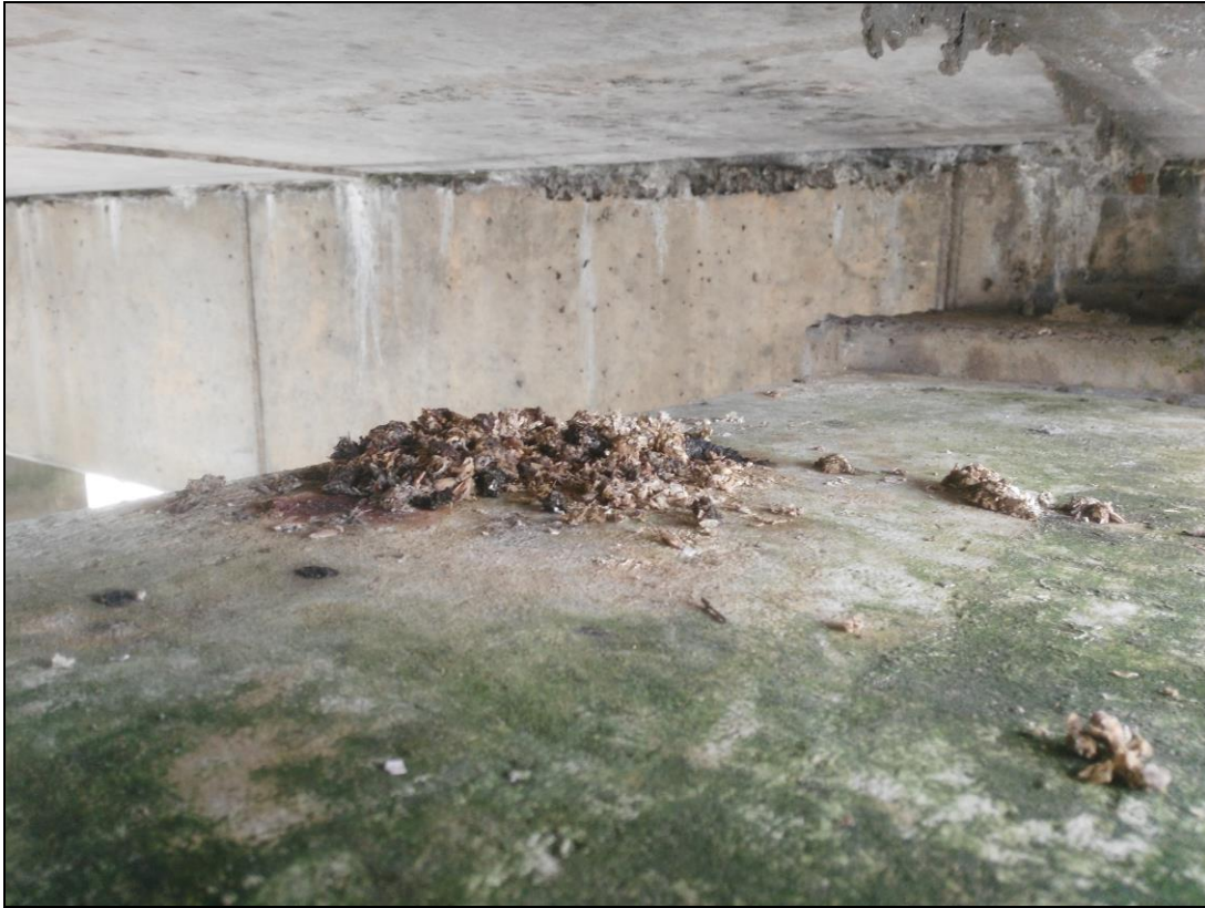
Plate 2. Accumulation of otter spraints recorded on concrete beam of pier structure during otter survey
