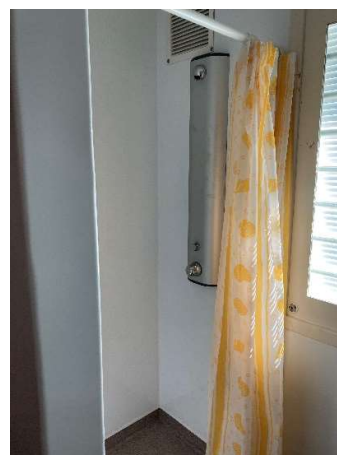
Figure 9: Shower in Isolation Room
