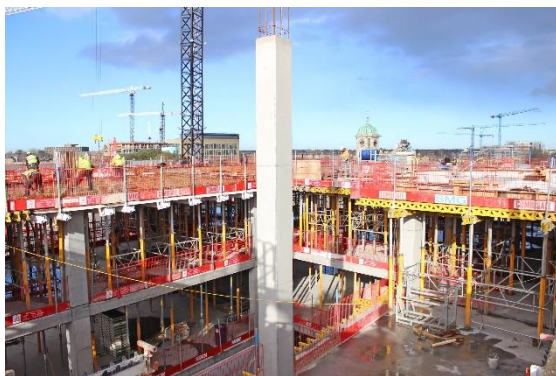
Construction of the East Quad, Grangegorman (photo courtesy of the Grangegorman Development Agency)
