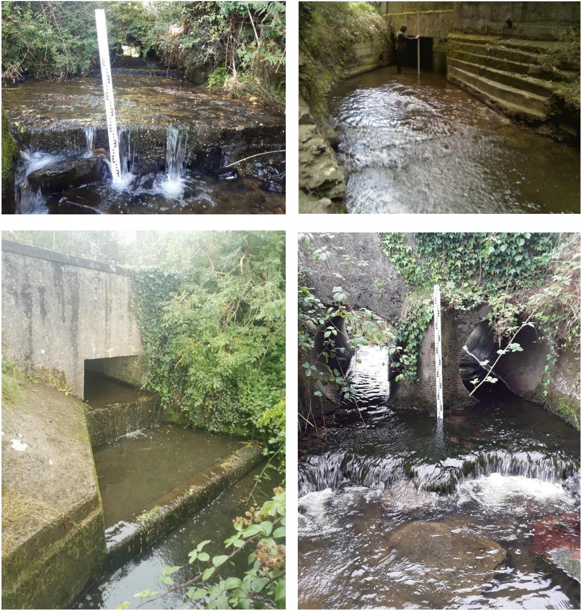
Figure 2.17 Examples of barriers identified during the Glyde survey, including two bridge aprons, a box culvert and double pipe culvert.
