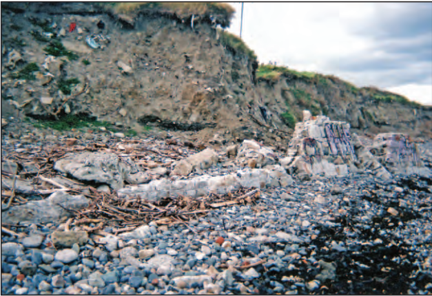
Plate 12.3 - View of consolidated ground with refuse inclusions and the remains of the embankment wall in the foreground, Landfall B
