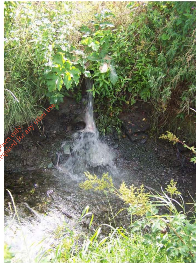
Above: Outfall from Ardfert WWTP into Tyshe River
