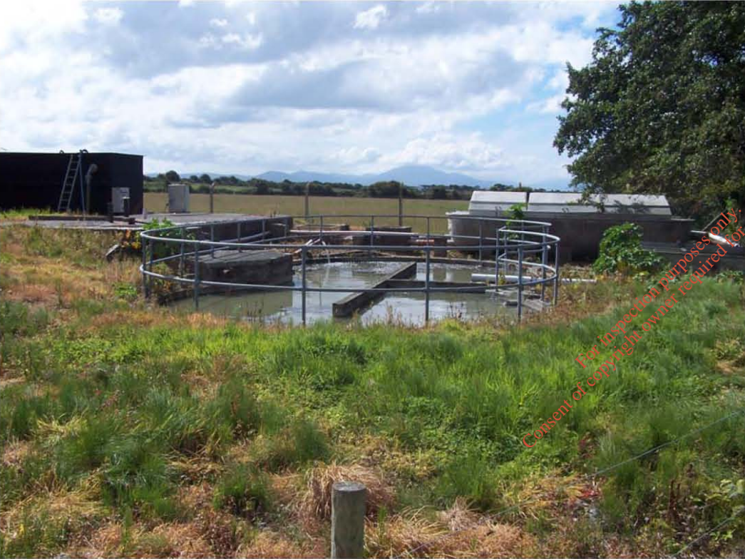
Above: Ardfert WWTP
