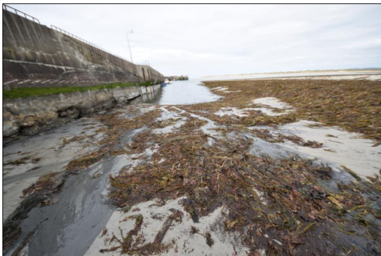
Plate 4 The subject pier. Water quality / visibility was poor and there was a large accumulation of rotting seaweeds. Sediments were anoxic.
