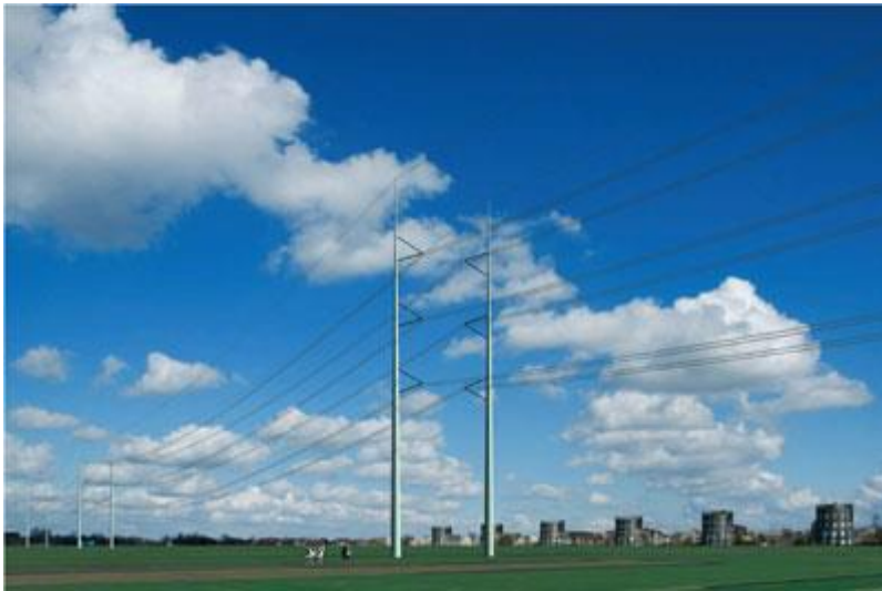
Figure 29: 'WinTrack' towers used for overhead line sections [44]
