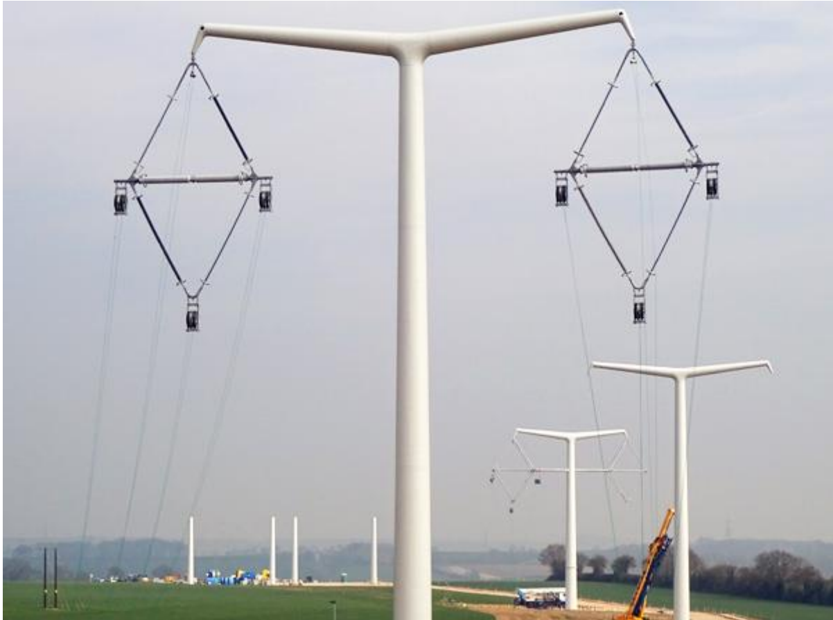
Figure 30: National Grid's 400kV T-pylon [48]
