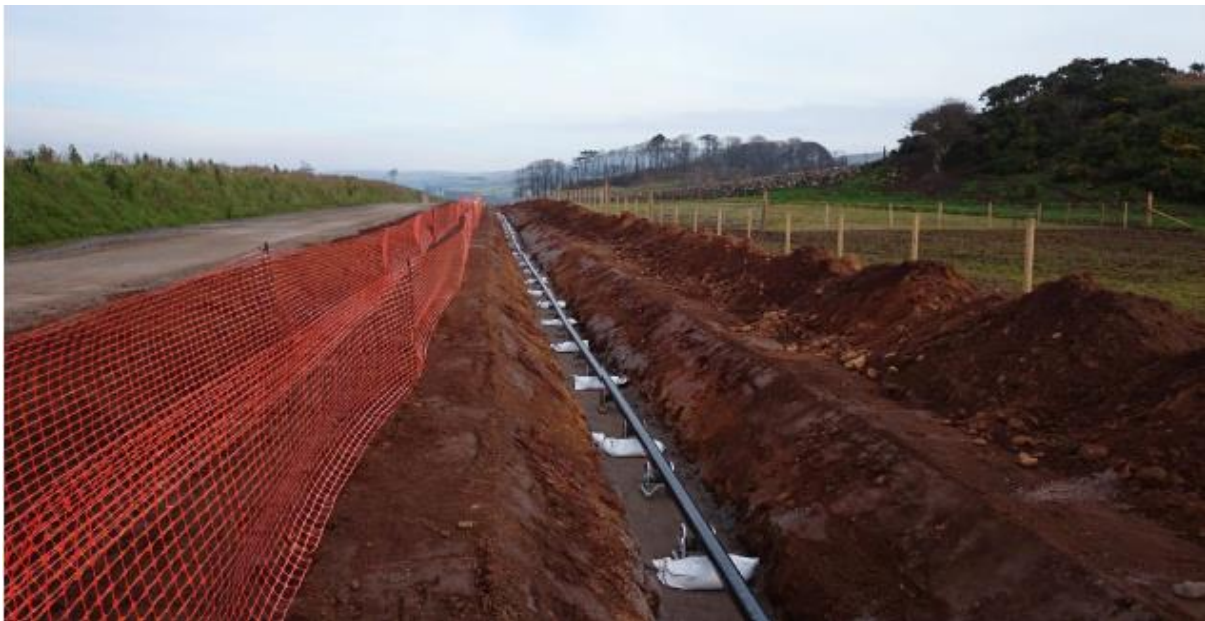
Figure 20: A section of underground cable under construction on the Western HVDC Link [36]
