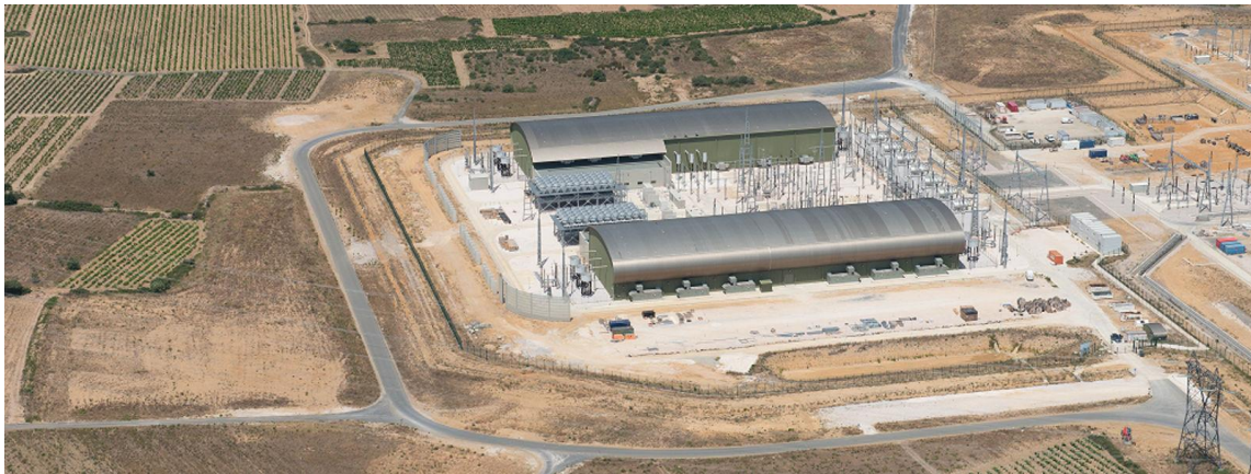
Figure 6: INELFE project: one of the converter stations [28]
