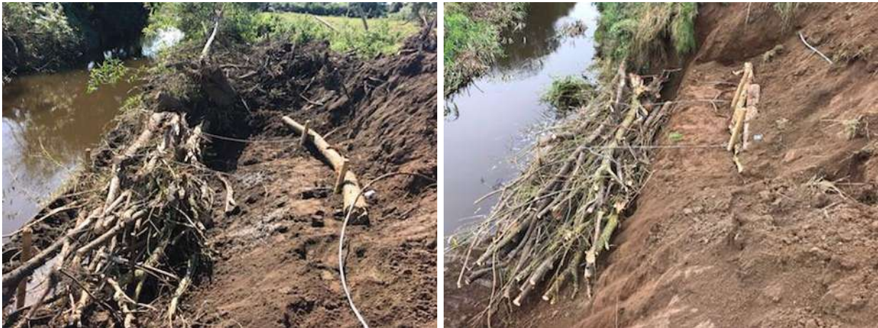
Figure 6.7 Soft engineering: willow bundles pinned to bank for reinforcement, which were then covered with a clay sod to incorporate the structure back into the bank.
