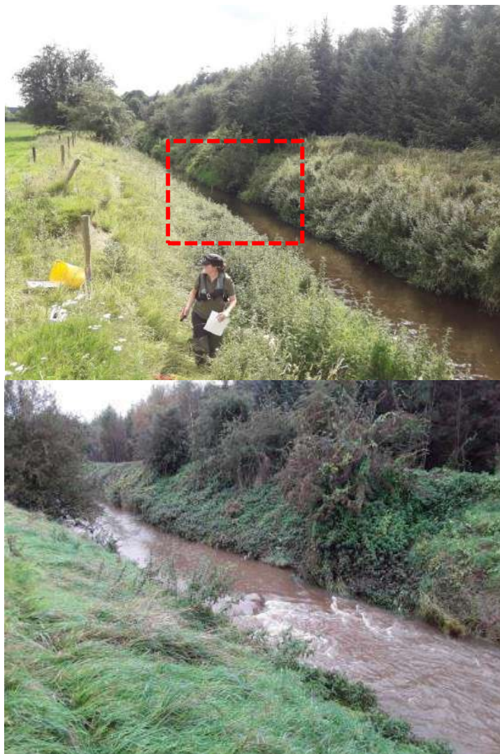
Figure 6.9 Example of pool excavation and riffle creation – before and after experimental digging.
