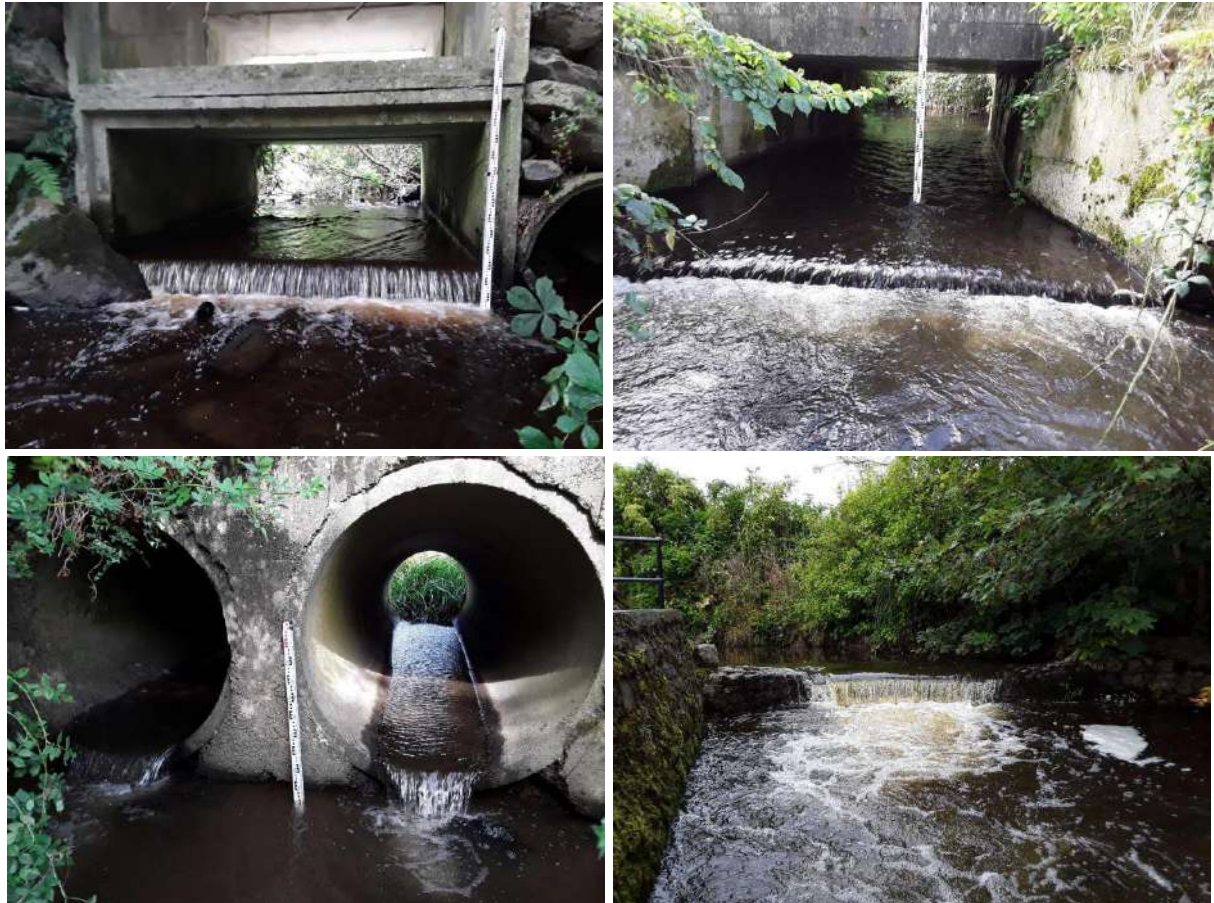
Figure 2.19 Examples of barriers identified during the Deel survey, including a box culvert, bridge apron, pipe culvert and small weir.
