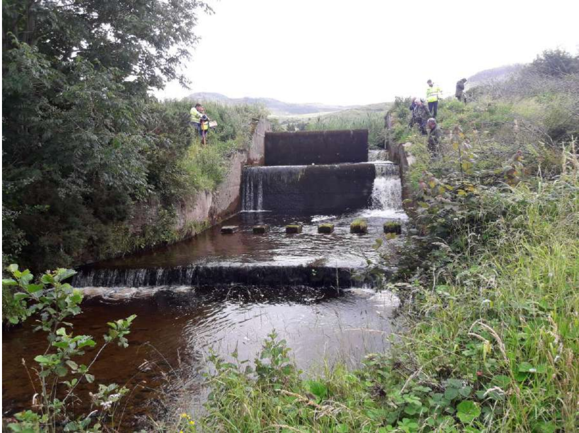
Figure 7.2 Gravel trap on the Largydonnell Stream, Duff catchment (ST8).
