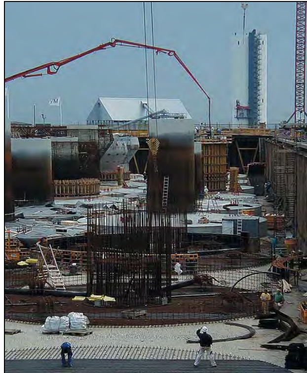
Figure 3.2 Concrete Gravity caisson foundations being fabricated for the Middelgrunden Project in Copenhagen Harbour.
