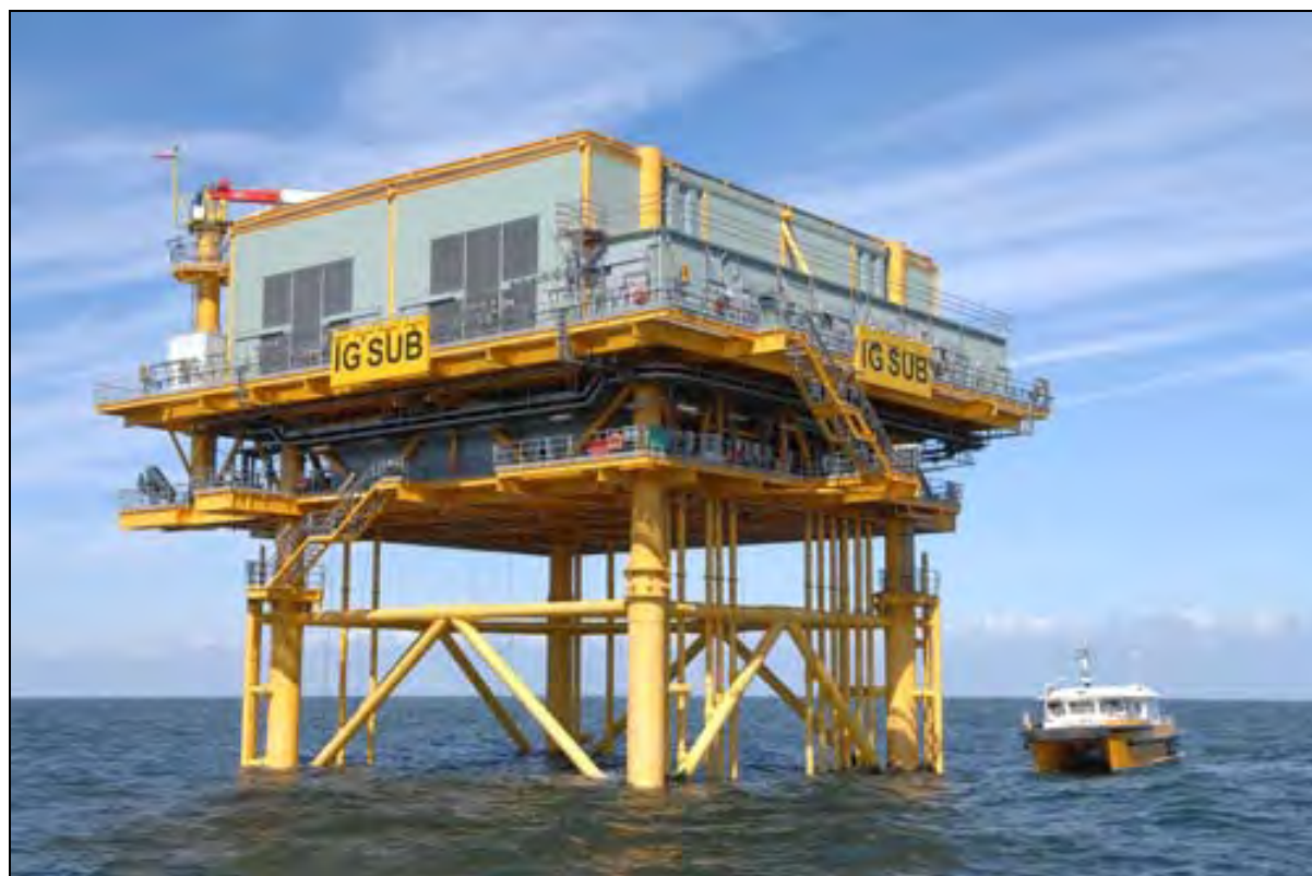
Figure 2.6 Typical Offshore substation
