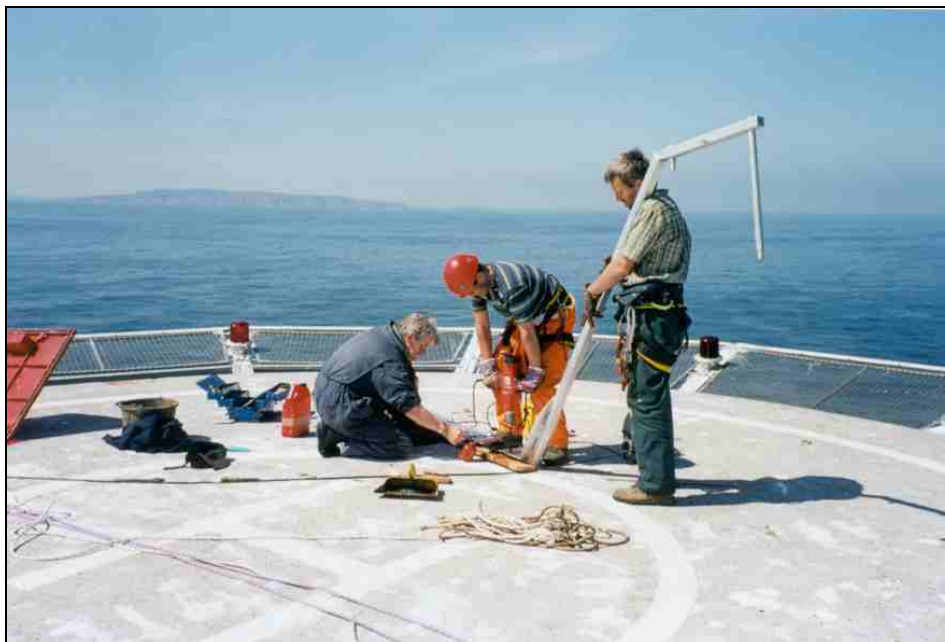
Figure 2.2 The installation of anemometry equipment on the Kish Lighthouse (courtesy of Irish Rope Access and Safety Consultants Ltd)
