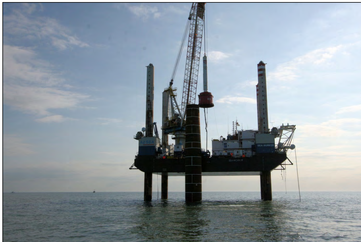
Figure 2.5 Installation of Steel Monopile at London Array Offshore Wind Farm (Photo courtesy of London Array Limited)
