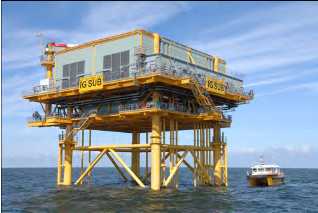
Figure 4.3 Typical Offshore Substation
