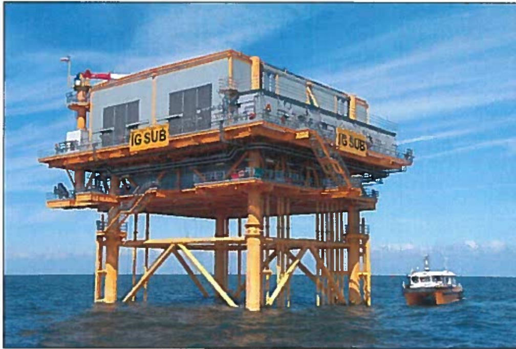
Figure 4.3 Typical Offshore Substation
