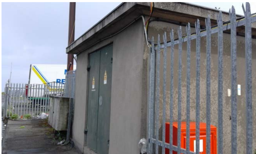
Plate 3: Substation present along the northern boundary of Zone A (Figure 3)
