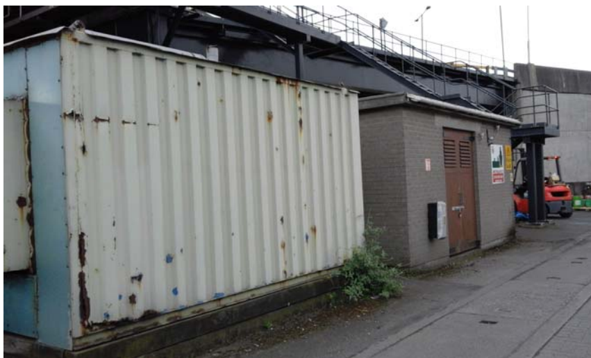
Plate 12: Substation/generator present to south west of Irish Ferries building
