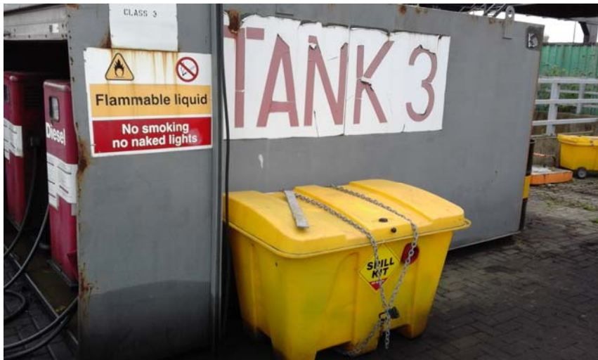
Plate 14: Fuel tank present to west of Irish Ferries terminal building with obvious staining of surrounding ground
