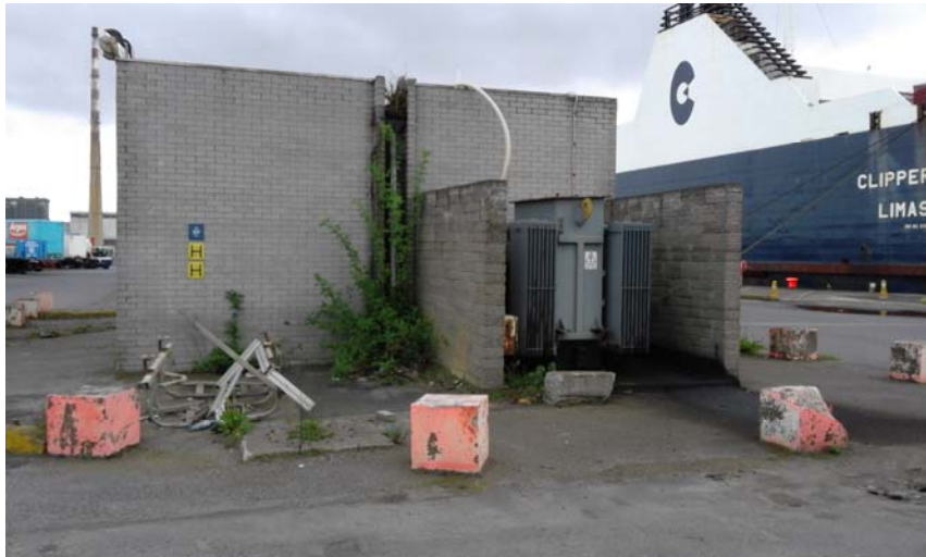
Plate 8: Substation present in southern portion of Seatruck terminal
